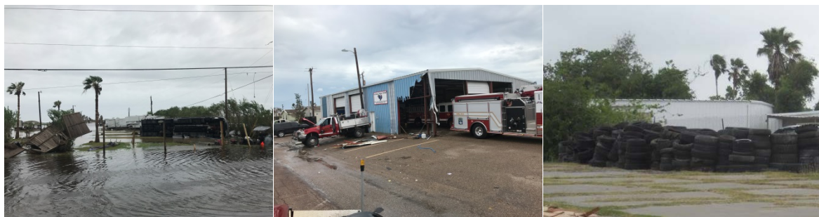
Figure 1. CS4-4. Water pooled in Port Aransas is a breeding ground for mosquitoes (left). The Port Aransas Fire Department roof is mostly intact, but the building sustained damage (center). Used tires in Aransas Pass (right).
